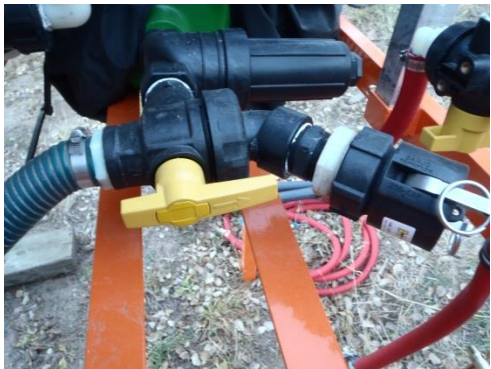
Source valve in fill position.
